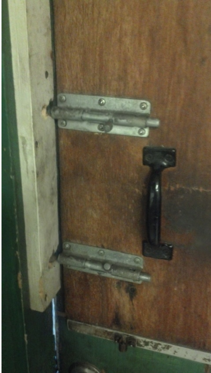
Slide Bolts -Unacceptable
